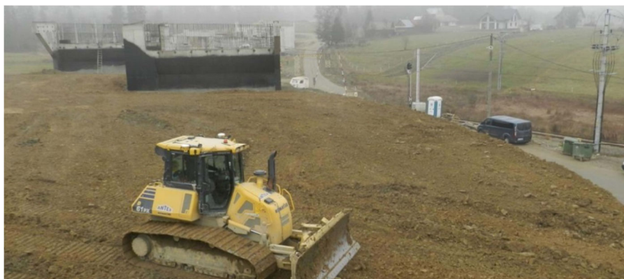
28. Nowy Targ bypass along DK 47 on the right line No. 99 in the area of the planned Grel branch post
