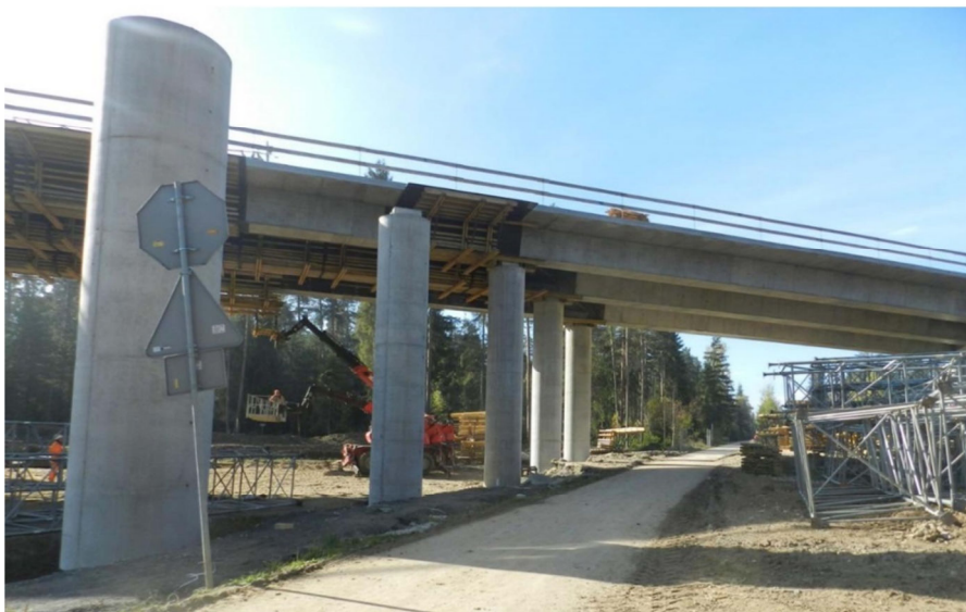
30. bicycle path, so-called Velo Dunajec running along the route of the former line No. 118 in Nowy Targ under the WD-121 structure of the Nowy Targ Bypass
