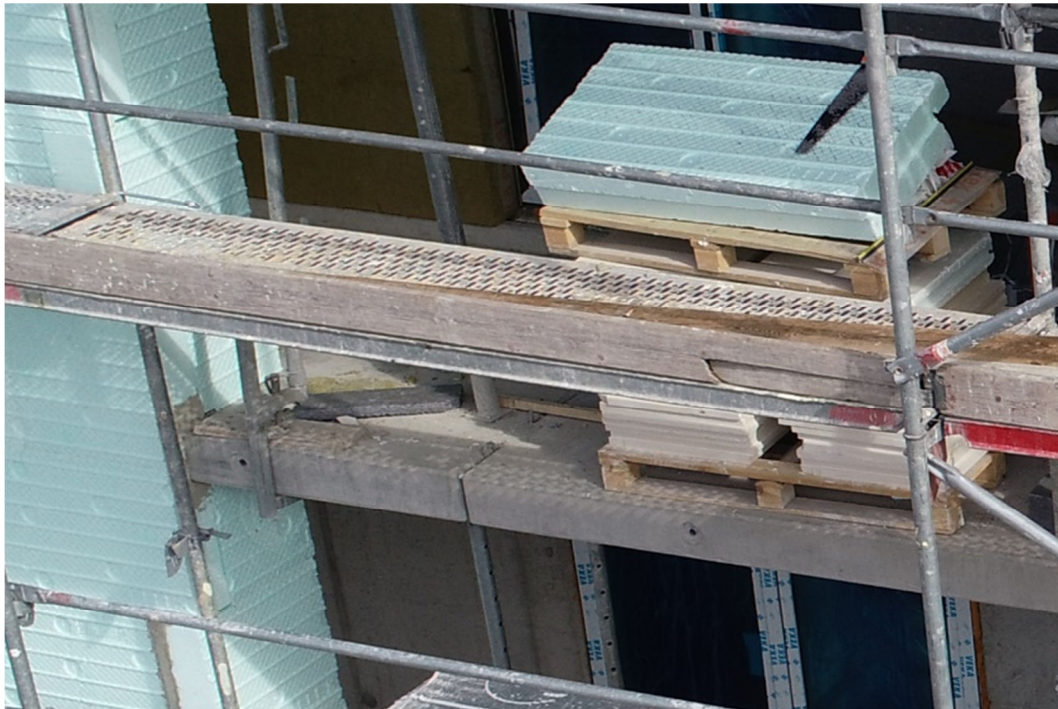
5. View of the damaged curb board
