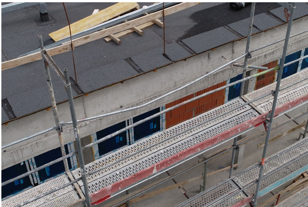
4. View of the damaged handrail
