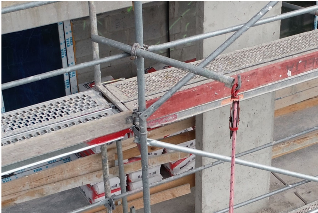
3. View of the winch
