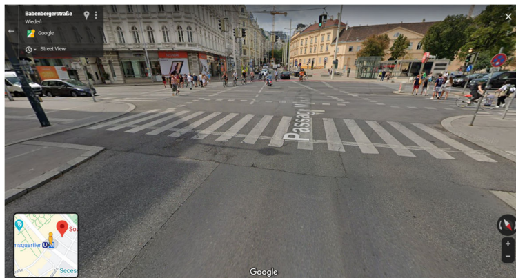
5. Leading lane made of chemically hardened masses - general view, Vienna/Austria (Photo: Google)
