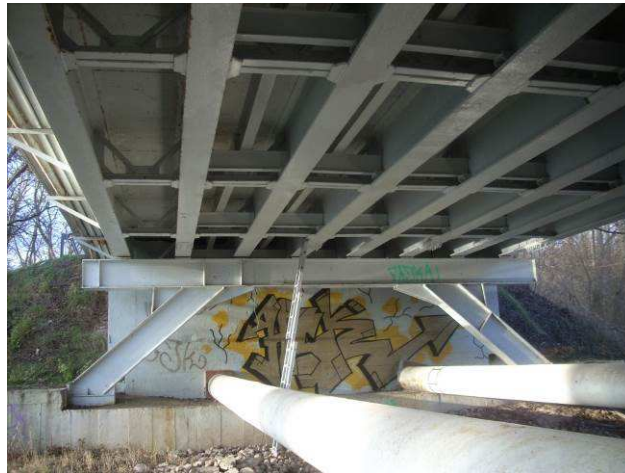
4. The construction of the bridge in the view from the underside of the span after strengthening
