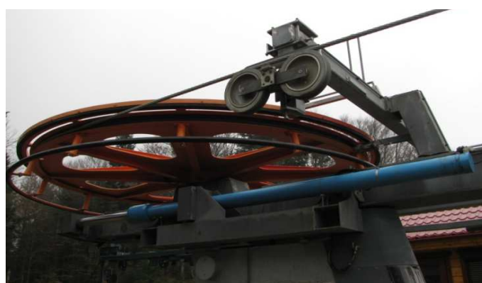
3. Hydraulic cable tensioning device "Słotwiny TAB" in Krynica Zdrój [6]
