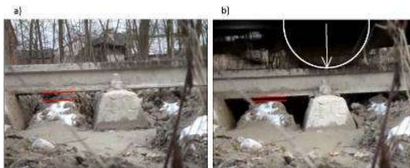
1. Deflection of rail track in the site of weak subgrade; a) the track without load, b) the track under load of rolling stock (visible reduction in gaps under sleeper) [22]
