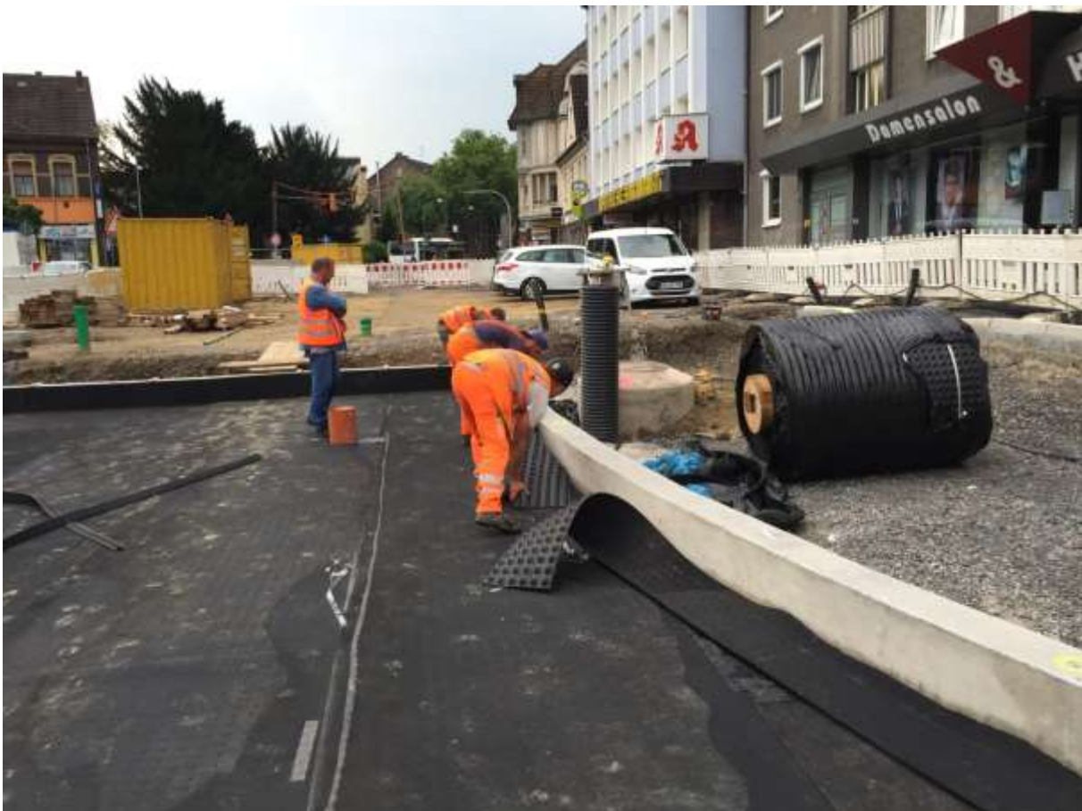
4. General view of the assembling mass - elastic: stage system: folding of vertical anti-vibration mat and connecting profiles, phot. Calenberg Ingenieure
