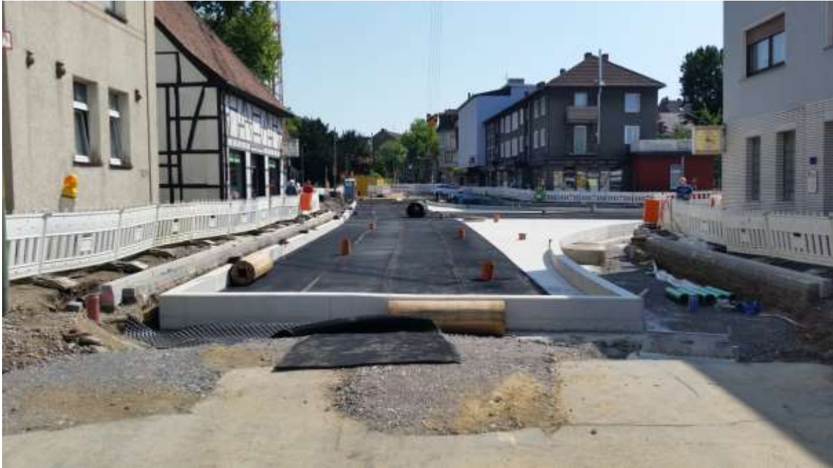
3. General view of the assembling mass - elastic system: folding of horizontal anti-vibration mat on a prepared surface, phot. Calenberg Ingenieure
