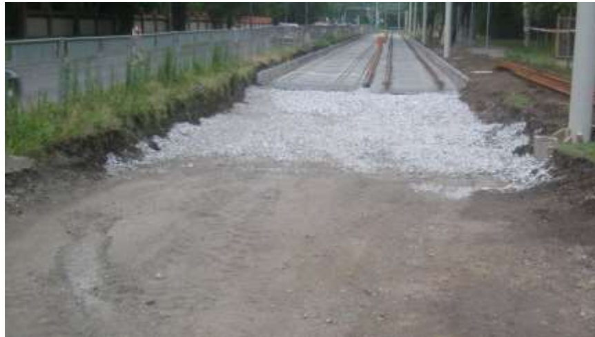
5. Solution of "sandwich" type with unsorted material as tight layer and drainage between tracks, under the classic unbuilt tracks (the street Grabiszyńska 2015)
