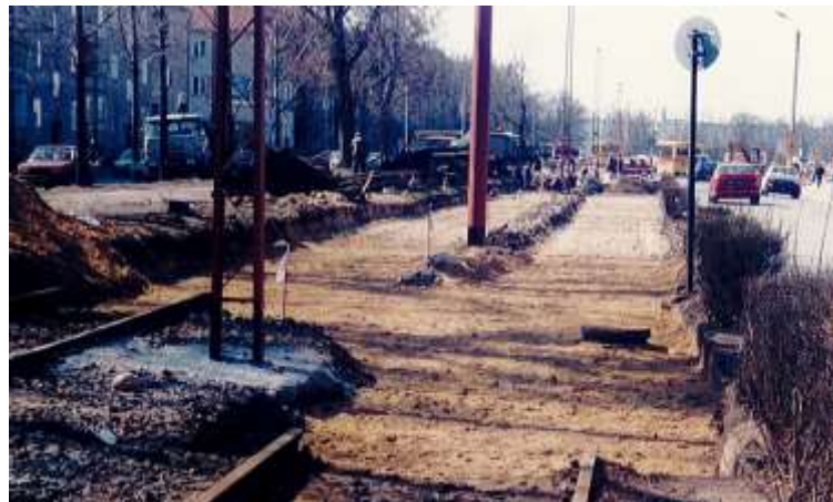
1. The solution of "just sand," under the classic unbuilt tracks (the avenue Hallera, 1997)
