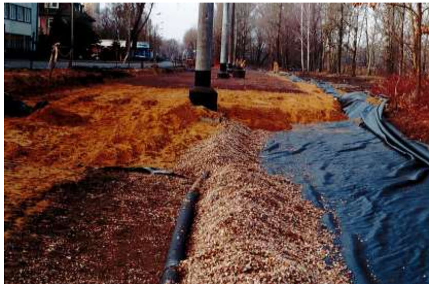
4. Solution of "sandwich" type with geosynthetics and drainage, under the classic unbuilt tracks (the street Kwidzyńska 2000)
