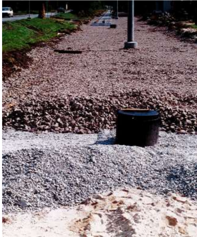
2. Solution of "sandwich" type with drainage under the classic unbuilt tracks (the street Lotnicza, 1998)
