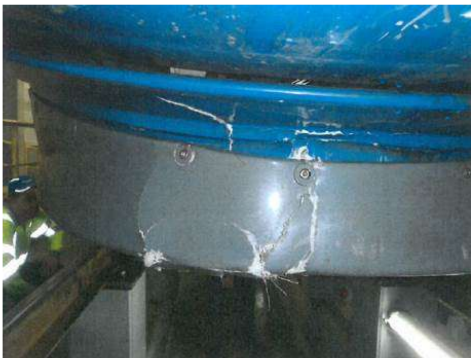
4. Cracked aerodynamic cover and scraper [Kałuża and others 2015]
