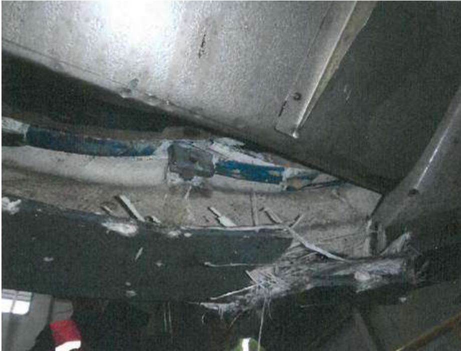
5. Damaged bottom scraper and cover of bow flaps [Kałuża and others 2015]
